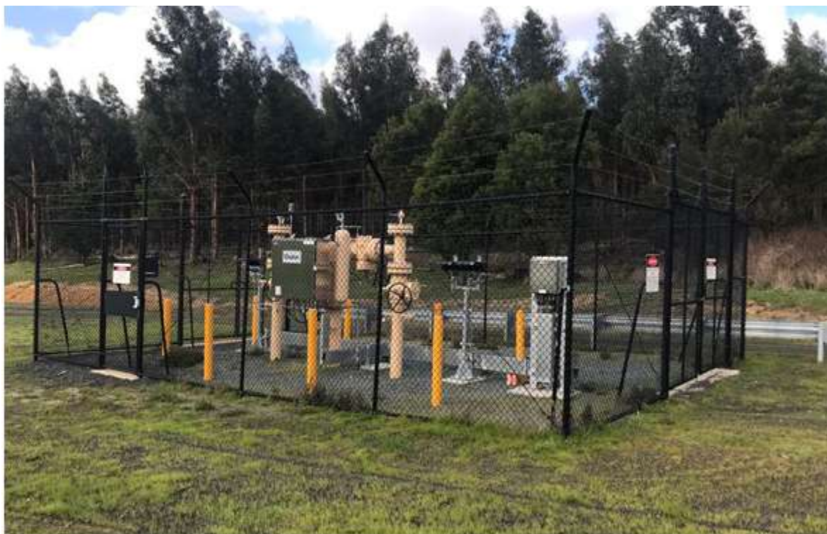
Figure 4 Typical mainline valve facility 19
